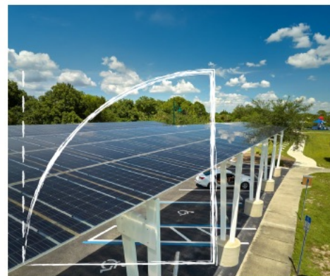
Ombrières parking photovoltaïques
